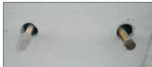
Figure 3.3.2 Neat finishes of installed services
